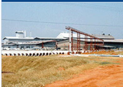
Construction work on a biogas pipeline, with the SWI facilities in the background
